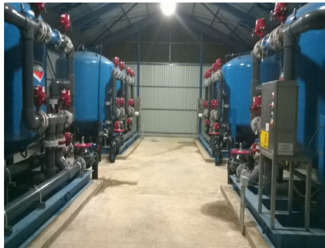
2.7 MGD arsenic removal system in Santiago, Chile using AdEdge's Bayoxide E33 adsorption media.
