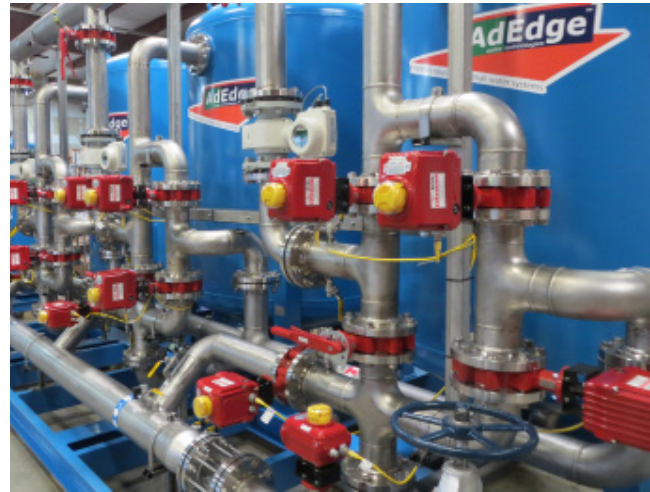
600 gpm manganese removal system in North Carolina using AdEdge's AD26 oxidation/filtration media.
