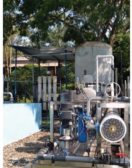
Figure 1: RO and UF system — UF system designed and constructed by Ecopolo ( www.ecopolo.co.br )
