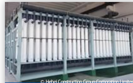
© Hebei Construction Group Corporation Limited Tratamento de Efluentes: 315,000m³/d
