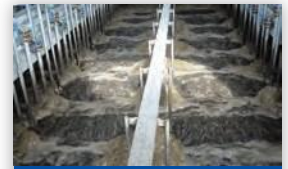
ETE Industrial : 10,000m 3 /d
