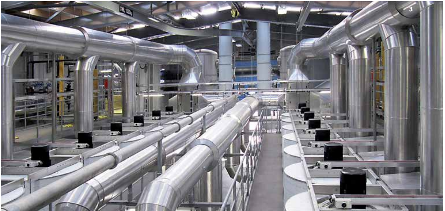
Air fans of two Low-Temperature-Dryers type Pro-Dry®
