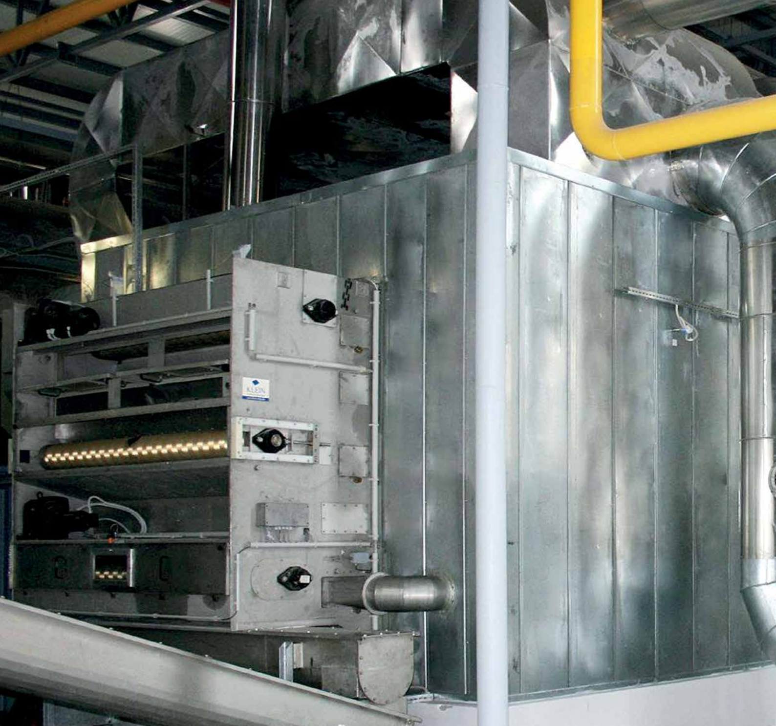
Pro-Dry® 3/5 (top), natural gas burner unit (center), distributor (right)
