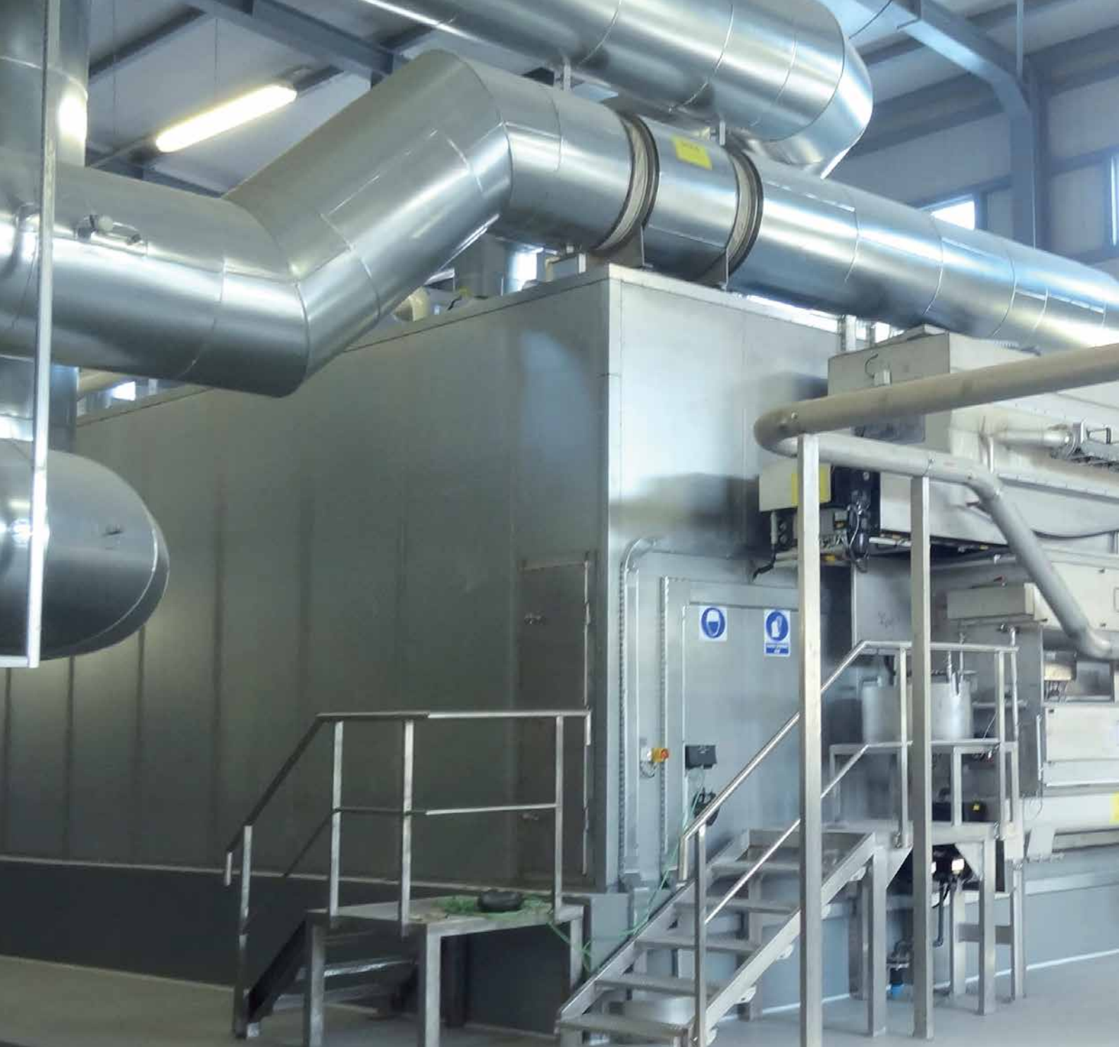
Pro-Dry® 2/4 (top), biofilter (center), sludge bunker (right)
