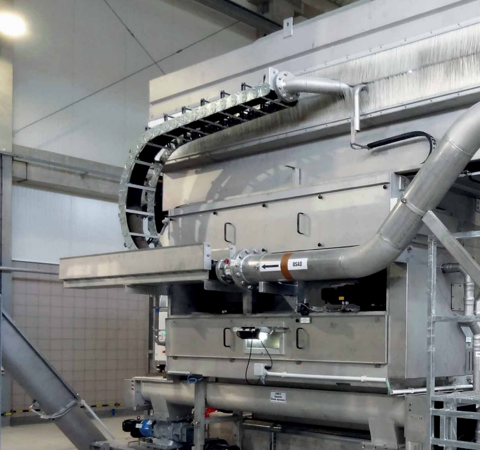
Pro-Dry® 2/3 (top), natural gas burner (center), sludge bunker (right)
