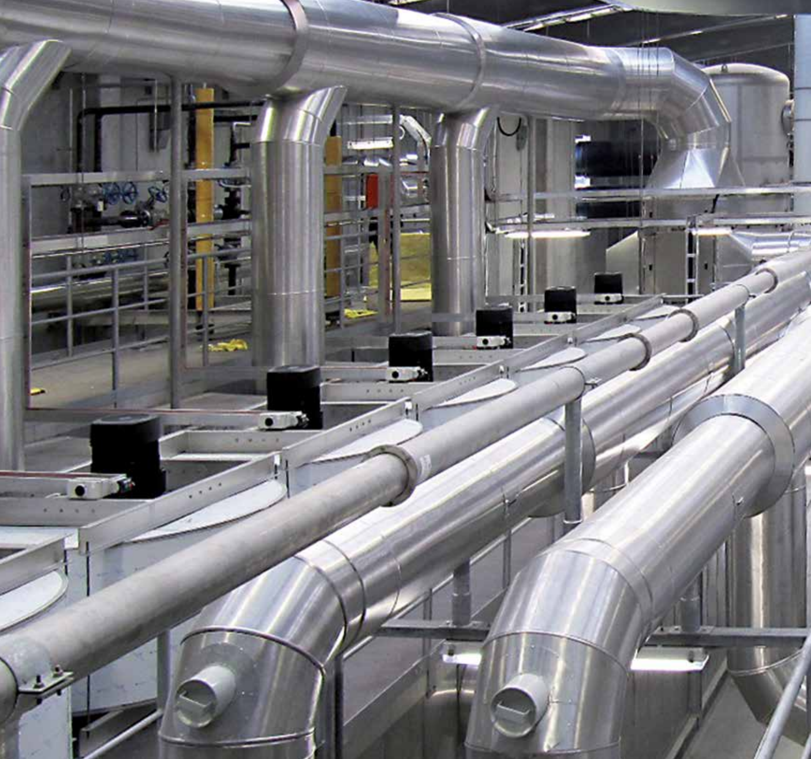
Air fans (top), two dryer lines (center), Pro-Dry® 2/4 (right)
