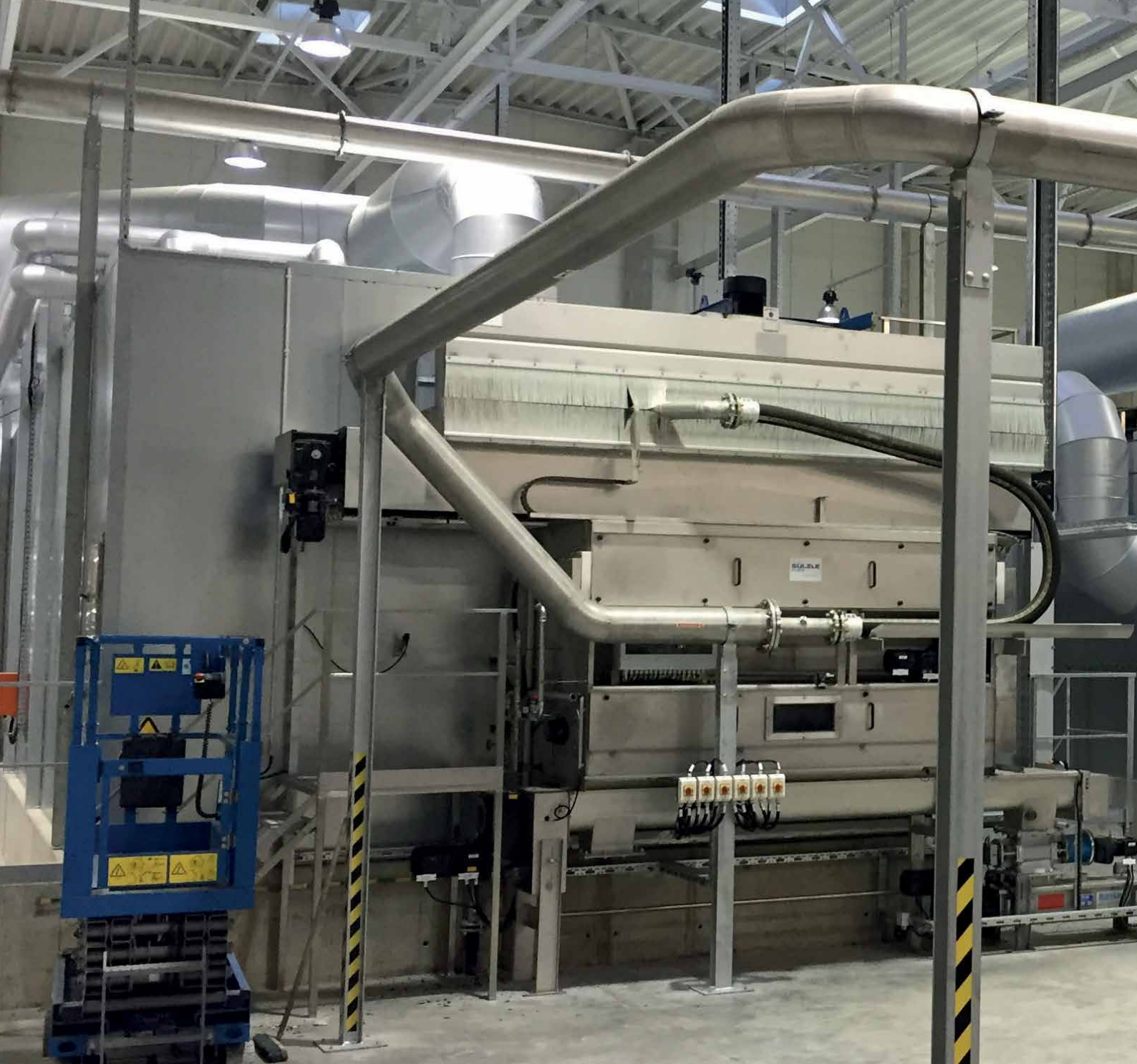
Two Pro-Dry® 2/4 (top), air fans (center), heat recovery (right)
